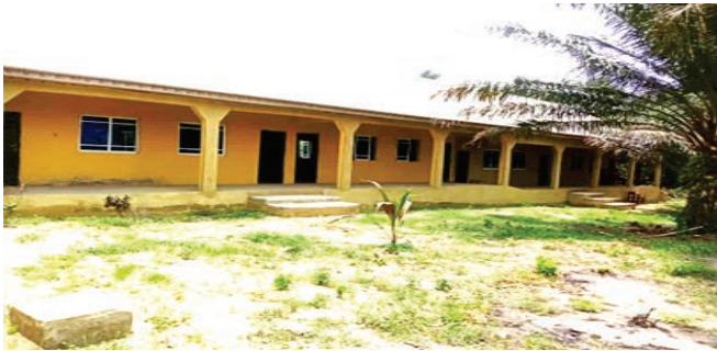
Block of four classrooms for Master of Divinity students under construction by Shepherdhill Baptist Church, Lagos.
